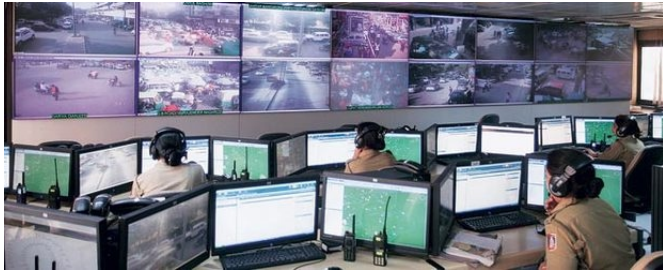
COMMAND & CONTROL CENTRE
